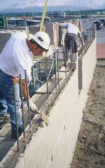
Figure 2. A new section of wall is getting started after grouting of the section below. The reinforcement being lapped extends into the next section of wall.
