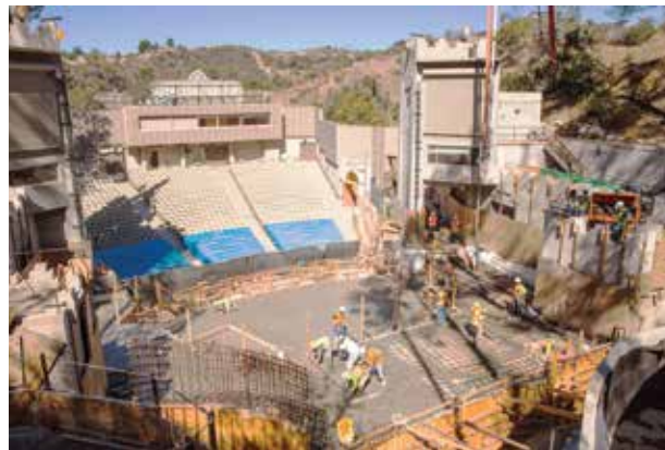
Figure 3. Construction of the new reinforced concrete stage. Courtesy of Levin & Associates Architects.
