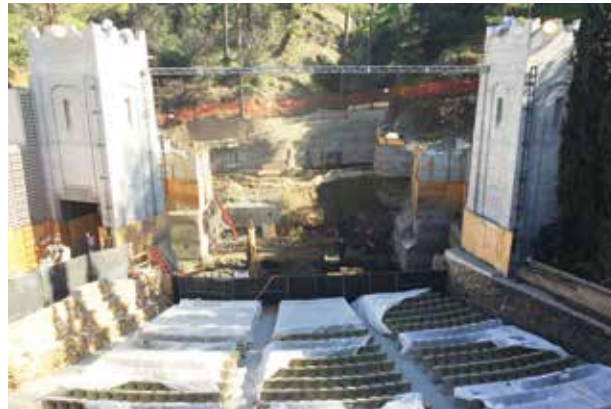
Figure 2. Construction of new stepped retaining walls behind the stage. Courtesy of Levin & Associates Architects.
