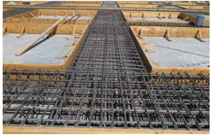
Typical jamb and header reinforcing and additional diagonal bars at inside corners.
