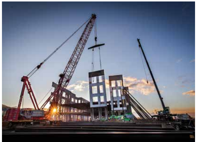
The Entrata Building is the first tilt-up building in Utah to be braced to the exterior during construction, using temporary bracing attached to temporary helical piers instead of the conventional deadmen.
