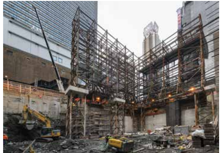
An as-built photograph of the existing structure and temporary support structure. Courtesy of Ralph D'Angelo.
