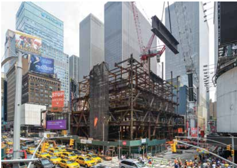
Erecting a 10-foot-deep plate girder for the seventh level transfer system. Courtesy of Ralph D'Angelo.
