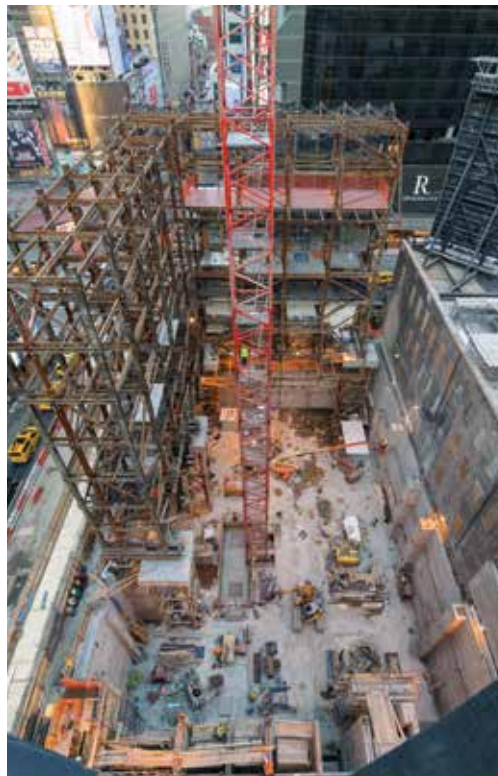
Overall view of the site at the completion of foundations. Courtesy of Ralph D'Angelo.
