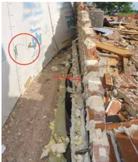
Figure 6. Damage consistent with previous tornado assessments – circle shows brick façade failure, arrow points to mortar buildup between bottom plate and brick veneer.
