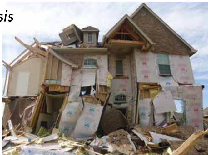
Figure 1. The March 2017 straight-line wind event took place in Rockwall, Texas, produced significant structural damage.
