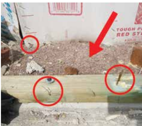
Figure 3. The flexible sheathing tore away from the bottom plate where staples were only partially embedded, allowing the balance of the wall to move inside (note that the arrow is pointing at the carpet).
