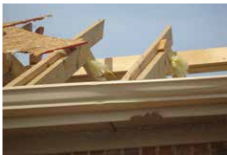
Figure 2. This roof had many staples oriented perpendicular to the rafter, and several staples had only one leg in the rafter.
