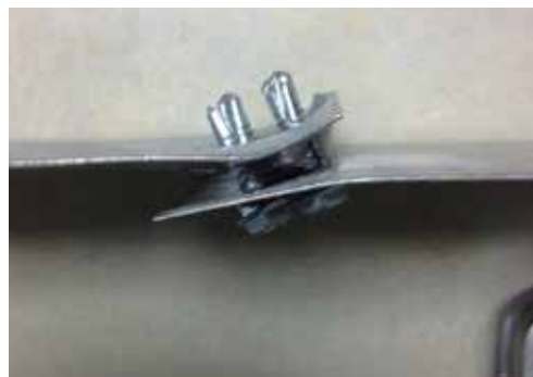
Gap between connected members.
