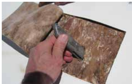
Figure 3. TPO roofing cut open. Decayed OSB roof sheathing cannot resist penetration. Courtesy of Ray Wetherholt.
