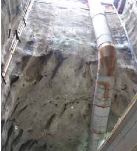
Figure 7. A view from the bottom of Shaft P (looking west) showing the tunnel access.
