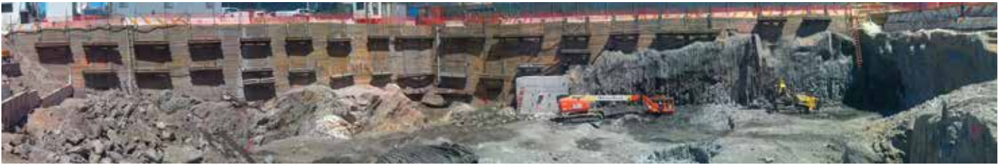
Figure 6. A view of the Northwest corner (towards the Javits Center) of the Phase II Soil SOE.
