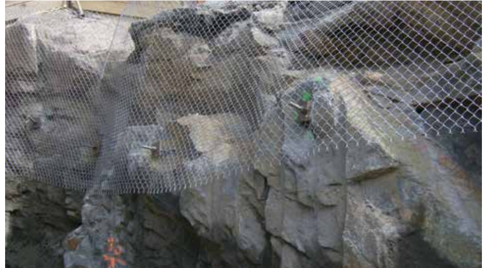
Figure 8. Typical rock bolts and mesh below the SOE.
