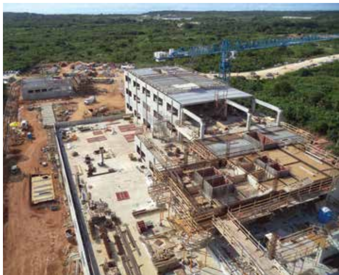
View from tower crane during construction. Courtesy of dck pacific guam, LLC.
