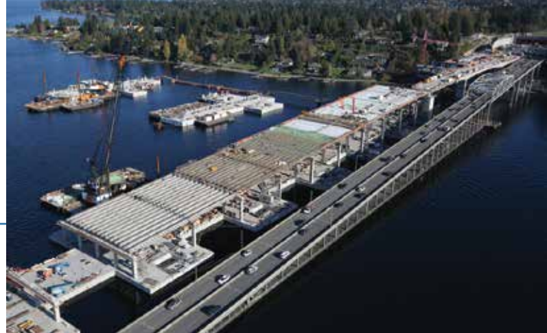
Aerial view of State Route (SR) 520 Evergreen Point Floating Bridge high-rise superstructure under construction.
