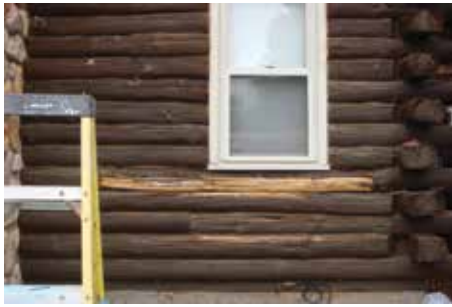
Figure 2. Close-up of rotten logs.
