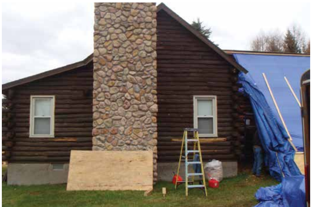
Figure 1. Elevation of deteriorated log wall.
