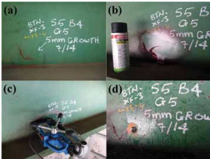
Figure 3. Fatigue crack arrest.
