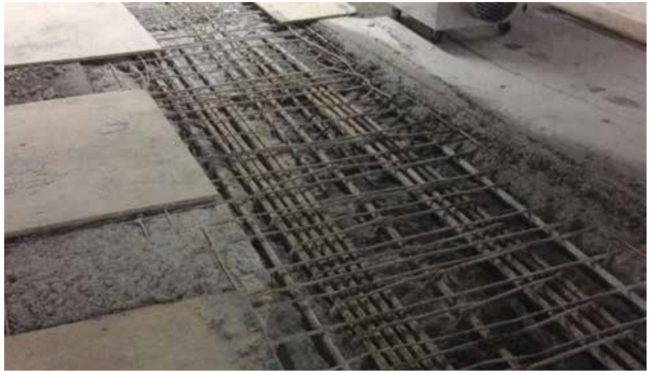
Congested reinforcing over a beam after demolition.
