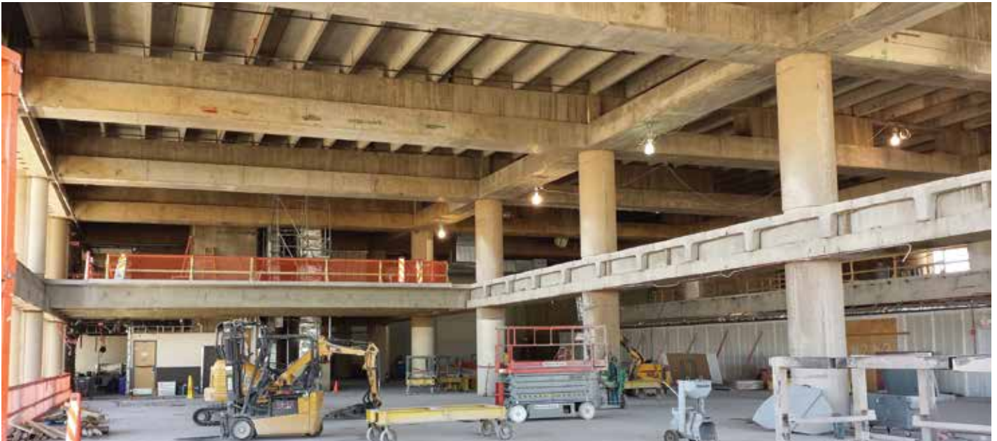
The building alteration included removal of large floor areas to create vaulted ceilings. These changes made significant impacts to the structural design of the building.
