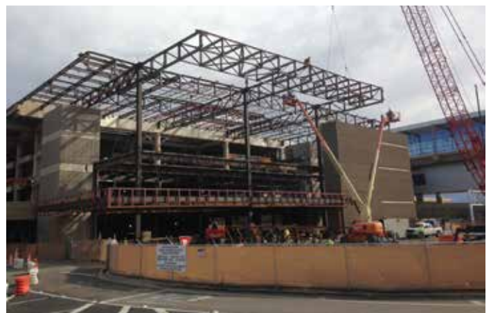
Structural expansion of the building adds 29,380 square feet of floor space. The steel structure attaches to the existing concrete, including a 37-foot cantilever.
