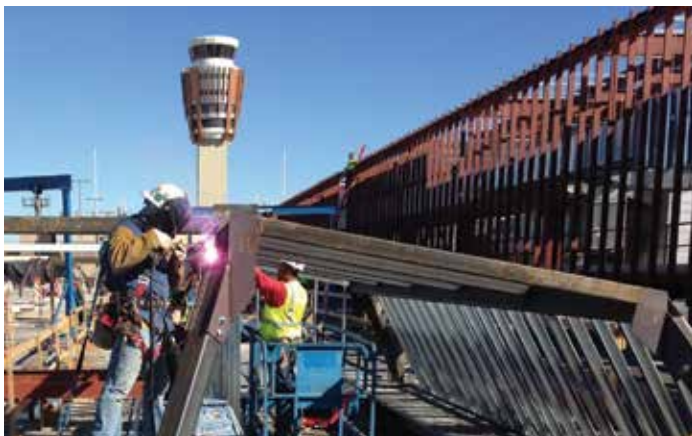
The addition of angled skylights diverts sunlight into the interior of Terminal 3. A welder puts the frame in place.
