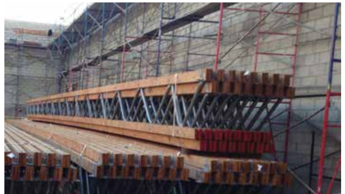
Figure 9. These single-piece 73-foot-long, top-chord-bearing parallel profile trusses will be installed onto wood-ledgers-connected concrete block walls.
