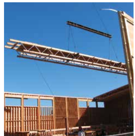
Figure 5. Spreader bar with proper pick locations lifted by a crane. Notice the second module in assembly jig on the ground.
