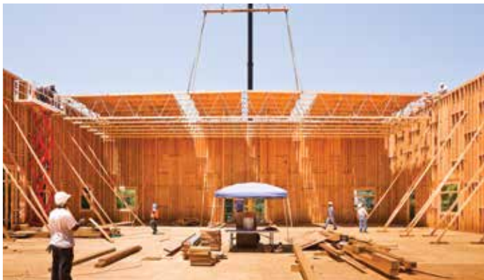
Figure 8. Modules of 89-foot-long pitched profile trusses for multi-purpose building hoisted into place by crane.
