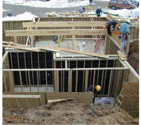
Properly designed, a PWF can be engineered with stress-graded lumber framing and plywood sheathing to support lateral soil pressures as well as dead, live, snow, wind, and seismic loads. Courtesy of the Southern Forest Product Association.
