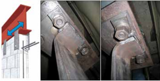
Figure 3. Original bent plate concept with non-ductile weld failure mechanism. Courtesy of International Masonry Institute, www.imiweb.org .
