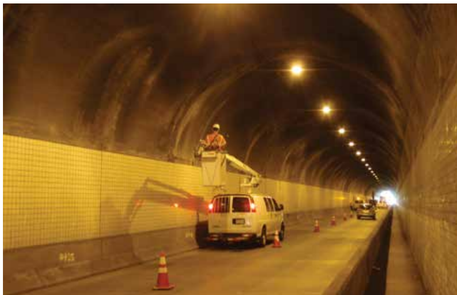
HDR inspector using a bucket van to access the arched concrete roof of a tunnel during a routine inspection.
