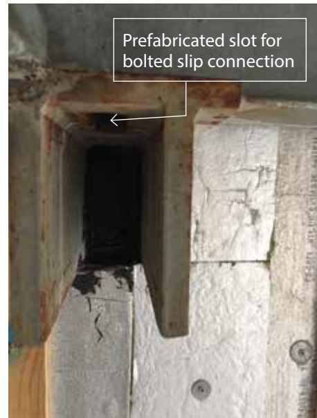
A pre-fabricated slot for a bolted slip connection. Note – just off the left edge of the photo are fillet welds of a bracket to the bridge structure.
