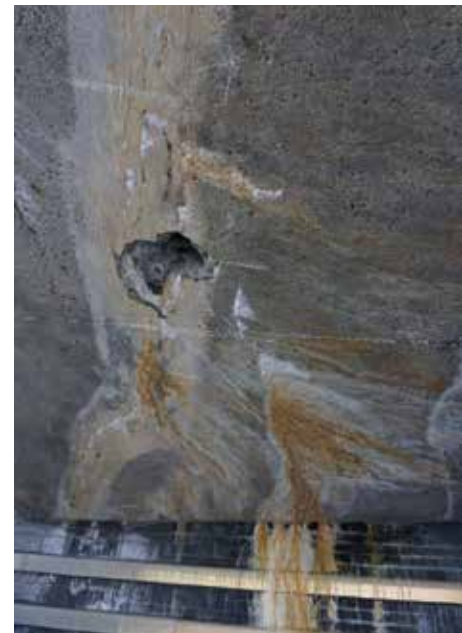
Figure 4. Efflorescence and water infiltration is visible on the south soffit of the cantilever.
