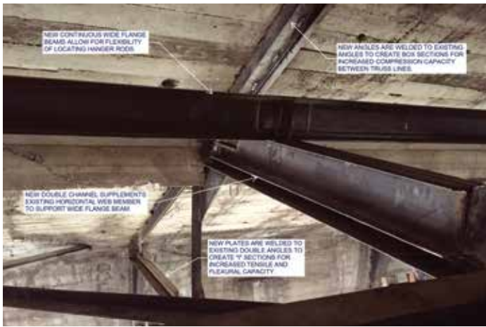
Figure 6. Construction photograph showing the modifications to the steel trusses needed to hang the rods.
