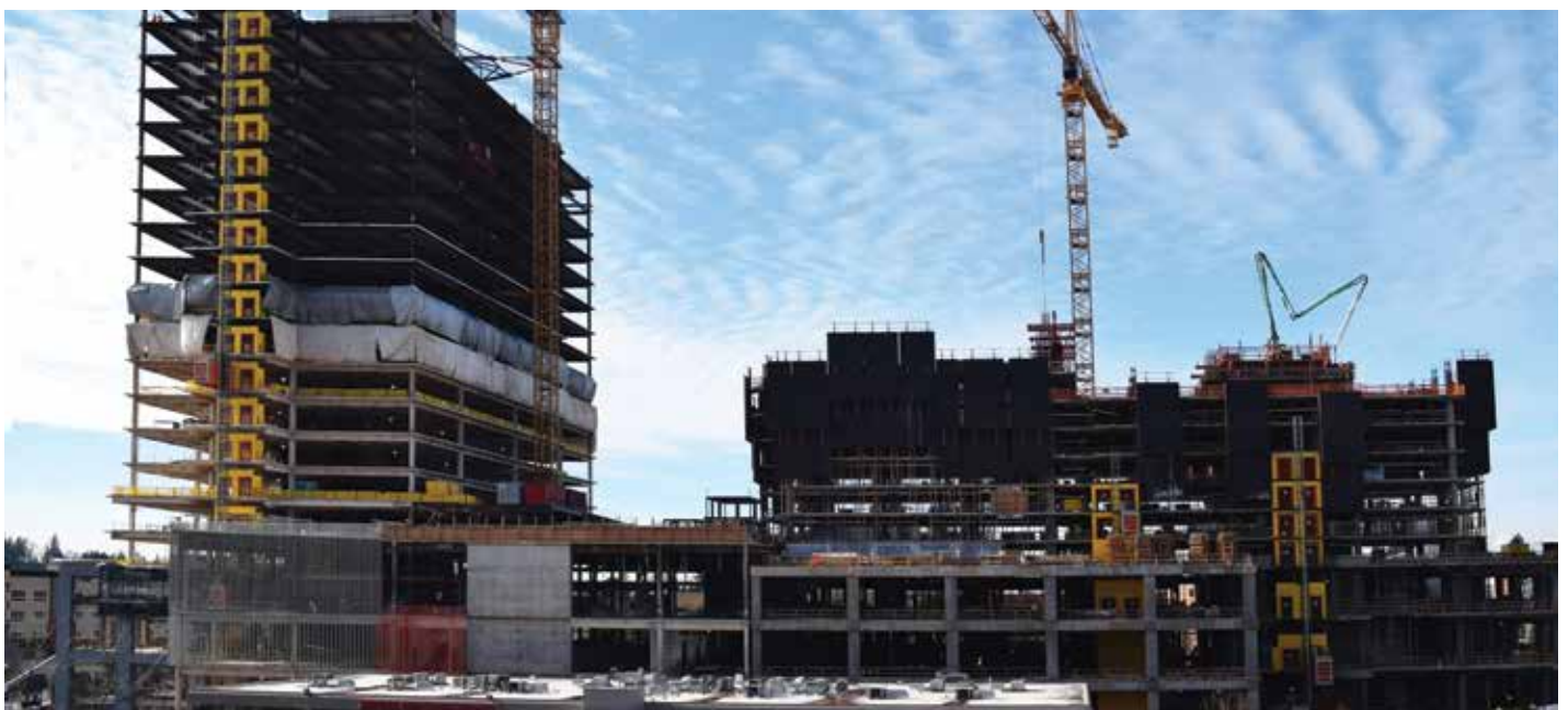
LSE under construction: steel office tower (left) and CIP concrete hotel/residential tower (right). Both towers will be 450 feet high.
