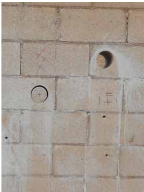
Figure 2. Illustration of the destructive nature of coring. The first attempt hit reinforcement causing further damage.
