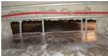
Figure 2. Existing slab is cut back to allow the FRP to be installed continuously from floor to floor.
