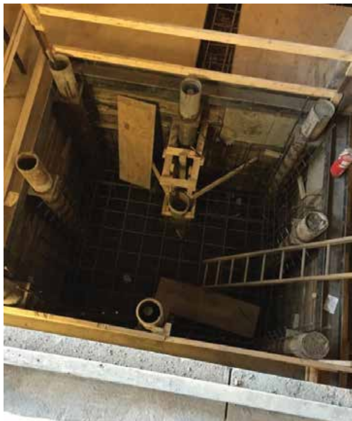
Figure 7. Aerial view of micro pile support of excavation at new elevator shaft.
