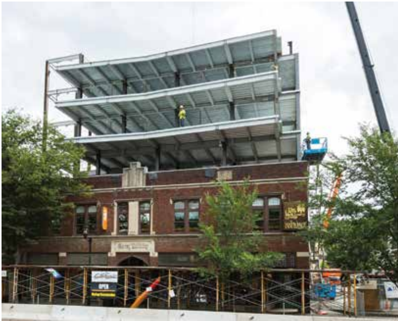
Figure 1a. Carey Building Southeast elevation during steel erection. Courtesy of Gary Hodges Photography.
