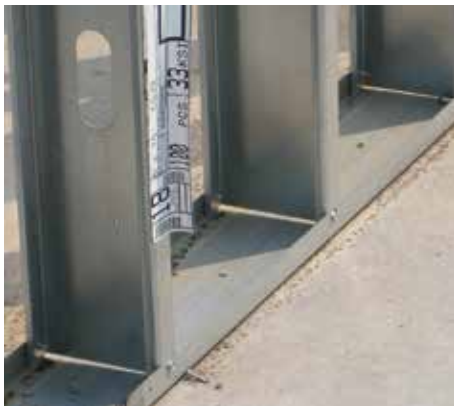
Figure 2. Nonconforming gap between structural stud and track.
