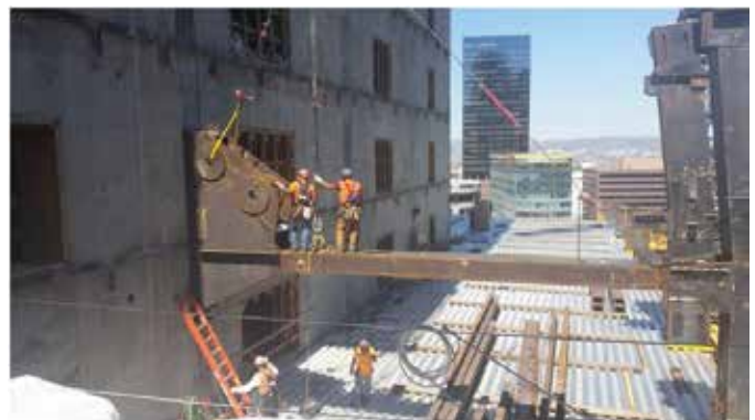
ESW-NG was recently used to weld BRB gusset plates to plates embedded in the concrete core of the Wilshire Grand Hotel in downtown Los Angeles.
