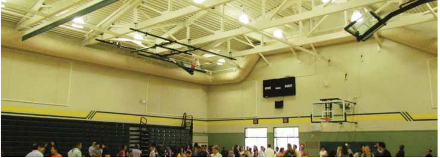
Figure 5. The cold-formed steel trusses and metal deck are part of the finished interior look.
