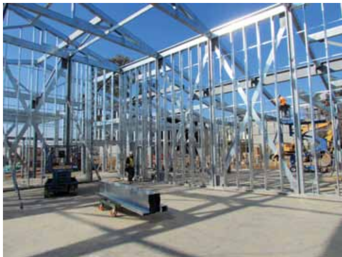
Figure 2. The HSS columns support the cold-formed steel trusses and are the “holddown” posts for the cold-formed X-bracing.
