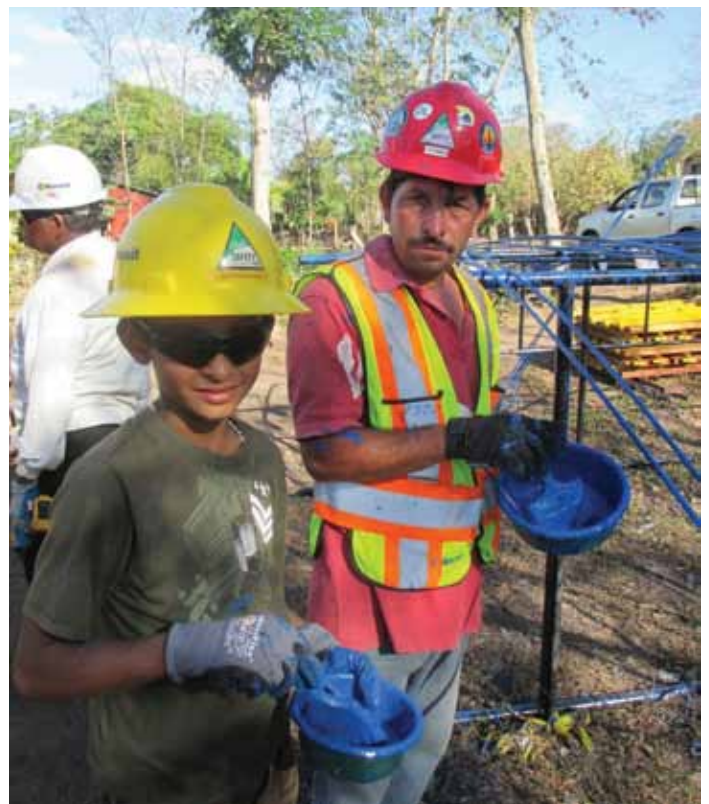
Fermin Garcia Espinoza paints steel bar hangers for the Rio Abajo footbridge. Courtesy of Ania Giffin.
