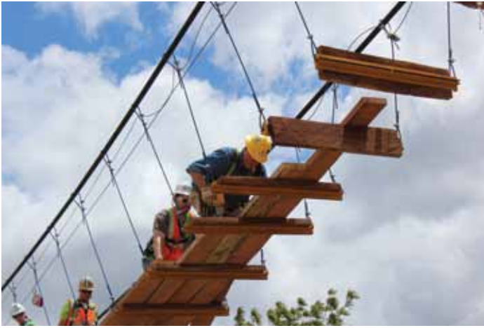
Build team members install deck planks made of tempisque, a local Nicaraguan hardwood. Courtesy of Abigail Conover.
