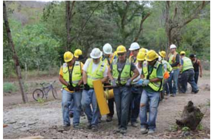
Community volunteers and bridge professionals team up to move the steel pipe towers. Courtesy of Abigail Conover.
