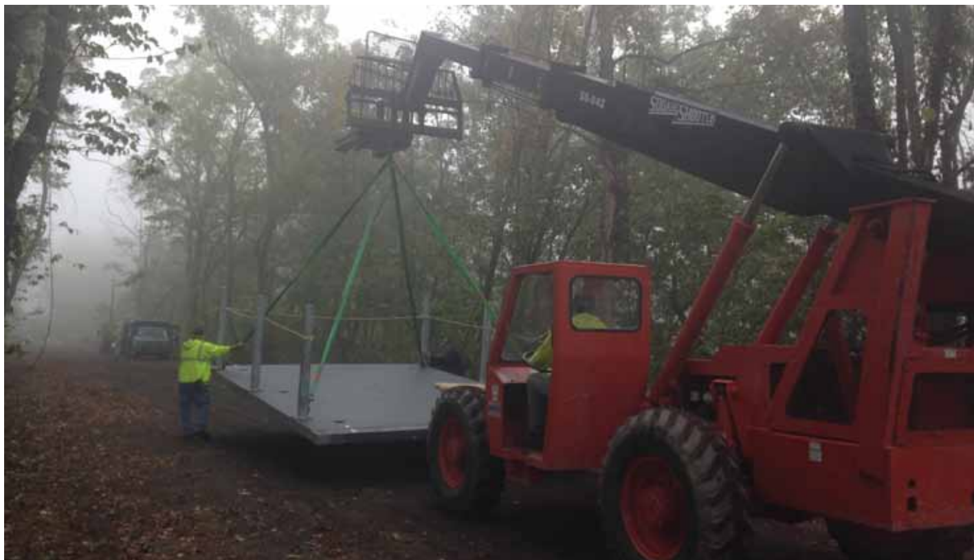
Figure 5. The lighter weight, high-strength FRP panels allow construction workers to maneuver FRP panels to the work site with just a telehandler.
