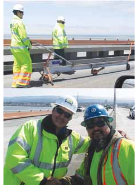
Figure 4. Top: Profilograph measurements ensuring contract compliance of quality ride. Bottom: Joint venture contractor foremen crossing paths in middle of bridge. One contractor worked eastbound lanes while the other worked westbound lanes.
