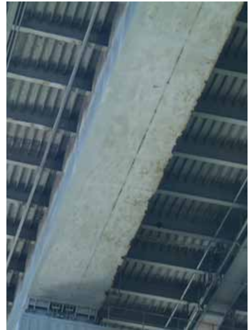
Figure 1. View from under showing ribs, girders and floor beams welded to deck plate.
