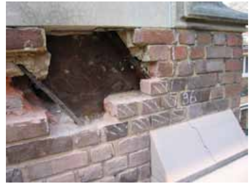
Figure 1. Cracking of masonry due to corrosion of the steel frame.
