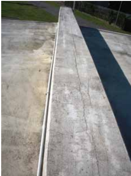
Exposed concrete deck and beams suffering from ASR. Area was patched 20 years ago and the lifetime of the patches has been reached. Waterproofing coating after replacing concrete surface would extend repair lifetime.
