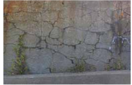
Typical look of a wall suffering from severe ASR damage. The failure is occurring due to the aggregate of the wall expanding and pushing out the outer layer.
