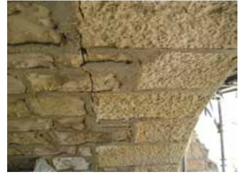
Longitudinal crack below spandrel wall, at junction with barrel vault.
