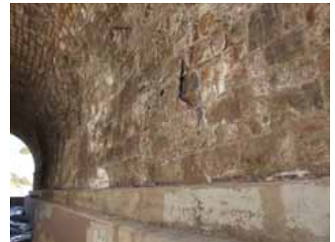
Stone spalling and deterioration due to freeze/thaw.
