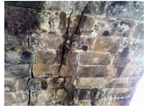
Large longitudinal cracks at stone arch intrados.
