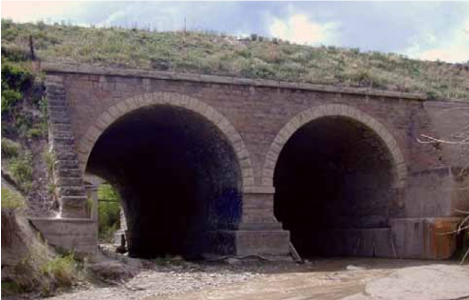
Two-span, stone arch bridge constructed in the late 1880s over Cottonwood Creek in Colorado Springs, Colorado. It served as a railroad bridge until the early 1960s when the tracks were abandoned. It was re-opened to vehicular traffic in 2012 after a restoration project.
