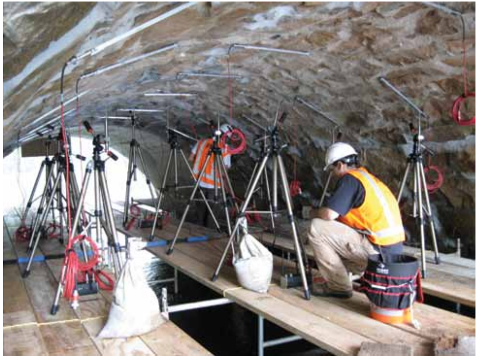
Typical live load test instrumentation layout, with LVDT sensors and strain transducers installed on the underside of the arch barrel.
