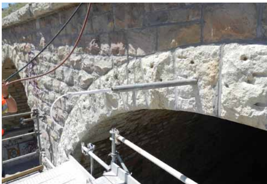
Grouted anchors used to connect a cracked (i.e. separated) spandrel wall to the arch barrel.
