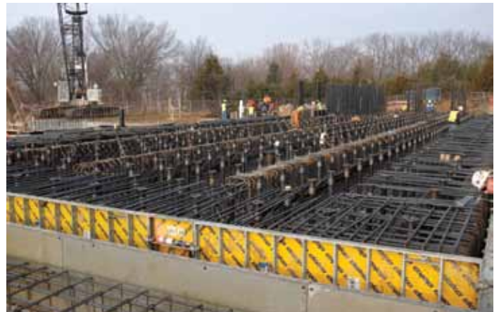
Figure 4. Strong floor with tie-down sleeves.
