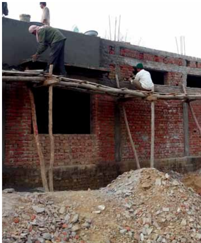
The issue was discovered only by viewing the construction photos as the plaster concealed the slab support condition.
