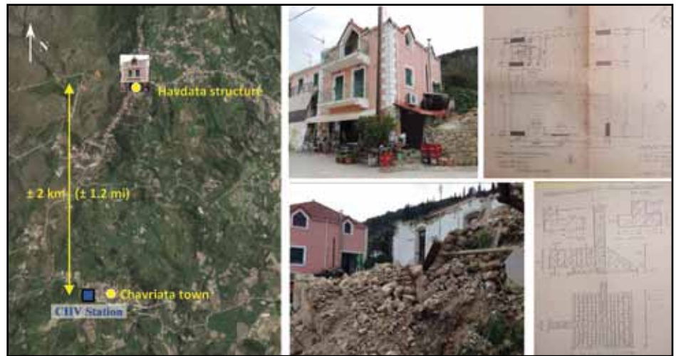
Figure 5. Havdata structure located 1.2 miles (2 km) north of CHV1 station sustained no significant structural damage while masonry building next to it collapsed completely. Copies of design drawings (right).
