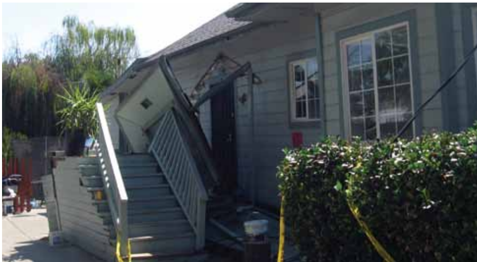
Figure 6. Residential cripple wall failure.
