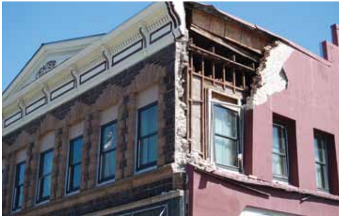
Figure 2. Damaged URM building.
