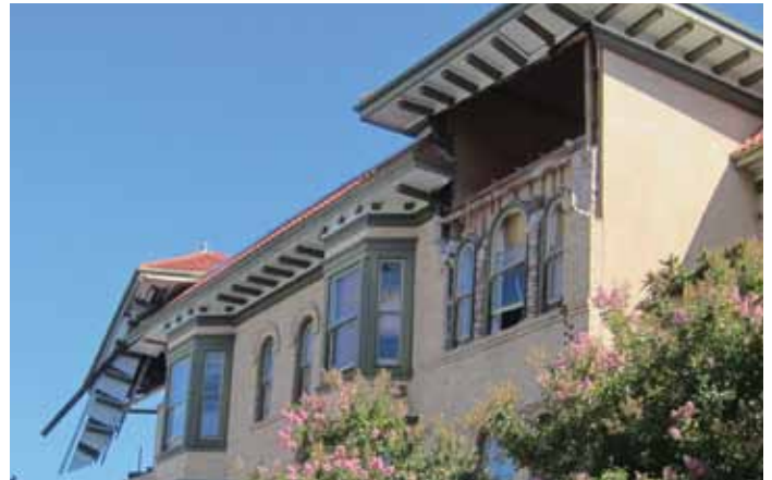
Figure 3. Damaged, retrofitted URM building.
