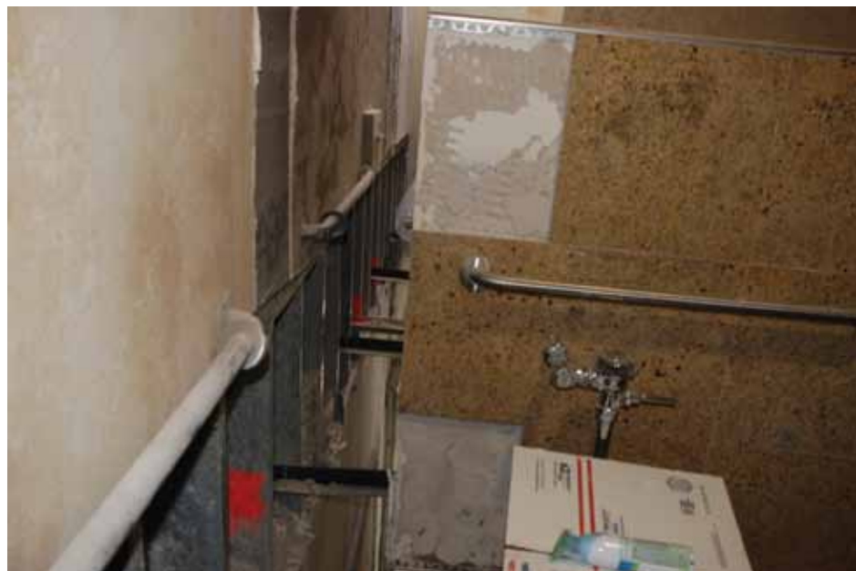
Figure 5. Exterior wall separation/gap.
