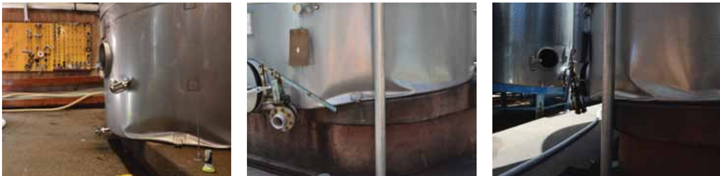
Figure 2. Damage to fermentation tanks. Examples of buckling of steel tank wall at base.
