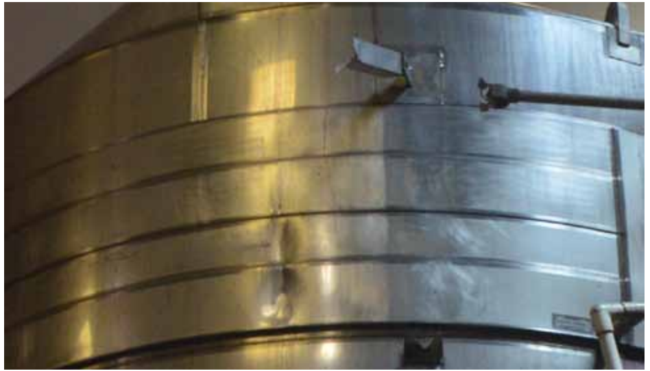
Figure 4. Denting of steel tank due to pounding of tank against catwalk.
