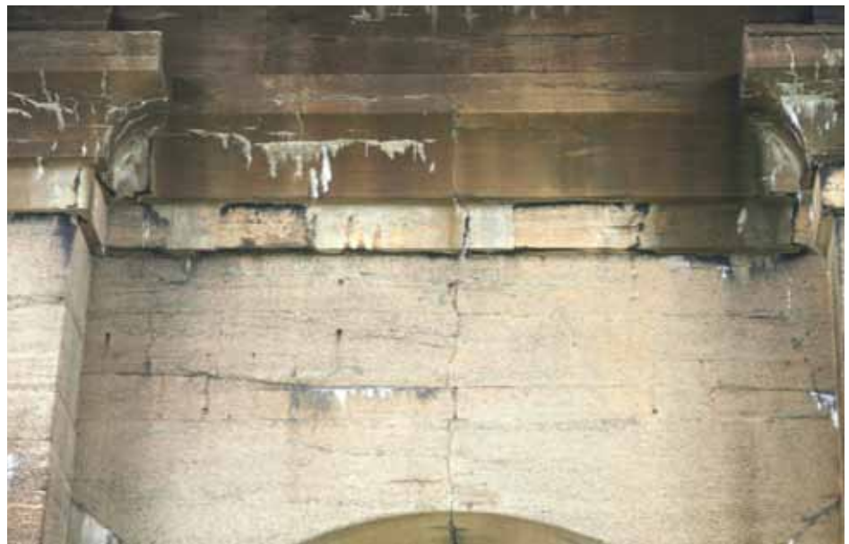
Figure 7. South face end pier 49. Vertical and horizontal popout-cracking, with ongoing severe spalling and alkali-aggregate reaction evident. New compounds from the reaction expand inside the masonry mass; the resulting localized pressure-zones result in microfracturing and spalling of the structure, here seen in the re-entrant spandrel-wall below the cornice. Cracks are oriented parallel to the bars. Volume changes and strength-loss of the masonry-mass are in progress.
