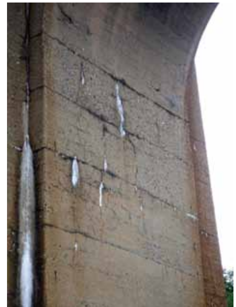
Figure 8. Cylindrical-vault abutment sidewall, end pier 53. Detail of active and desiccated white alkali deposits from reactions between inherent chemicals in the cement and aggregate, thermal effects, polluted air, and moisture. Note the resulting pattern-cracking below the arch springing. Increasing permeability of the mass and incipient oxidation of reinforcement are contributing to the cracking.
