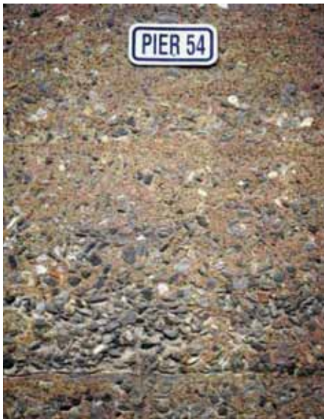
Figure 6. East face, pier 54. Permeable, century-old weathered concrete surface with exposed, large-sized aggregate which appears to have settled at the time of the pour. Note the one-part Portland cement to one-to-two parts fine-aggregate mortar slushing-edge between the horizontal pour layers. AREMA 1911 Specifications, in use at the time, stated that a uniform distribution of materials shall be obtained with the use of a straight slicing shovel after each pour.
