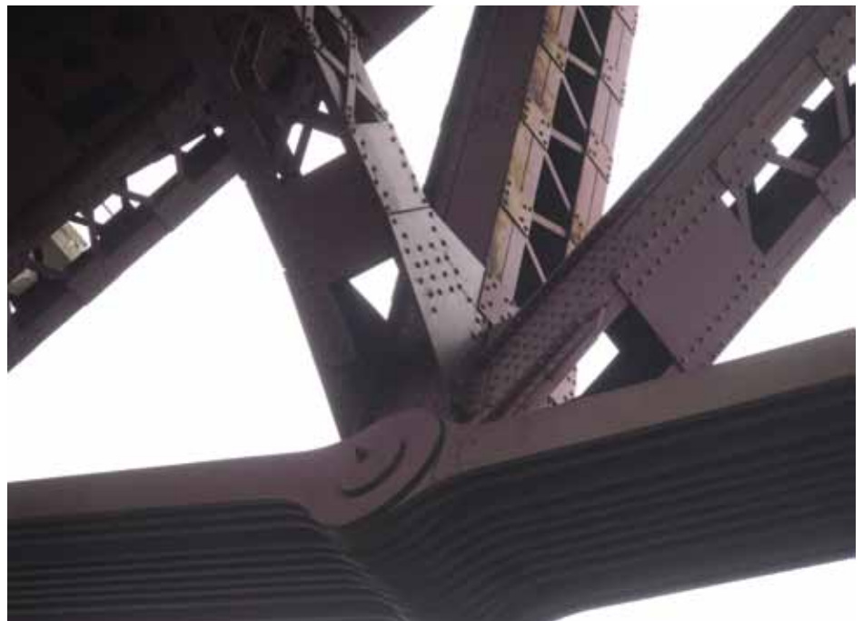
Figure 5. Detail, Little Hell Gate Reverse Bowstring Truss Bridge, 1915. Lower tension chord of eye-bars, with a view up to the deck, illustrating an array of structural steel truss members. Except for the eye-bars' 16-inch diameter pins, the bridge is riveted to exacting specifications, at the high cost of 25 cents each.
