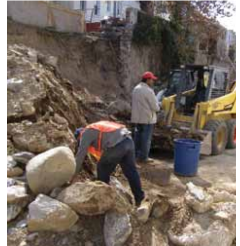
Figure 5. A visual inspection prior to collapse might not have detected that the wall was only 2 feet deep.
