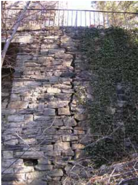
Figure 1. Crack in rubble wall.
