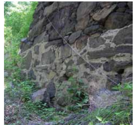
Figure 6. Collapsed dry wall. Repair pointing at the base, intended to keep pins in place, might have contributed to collapse.
