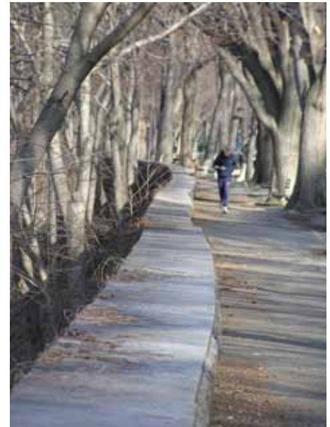
Figure 3. Irregular alignment at top of wall.
