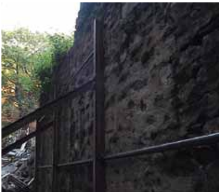
Figure 2. Retaining wall stabilized with rakers after collapse. Note lean of wall.
