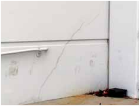
Figure 4. Cracking associated with base restraint.
