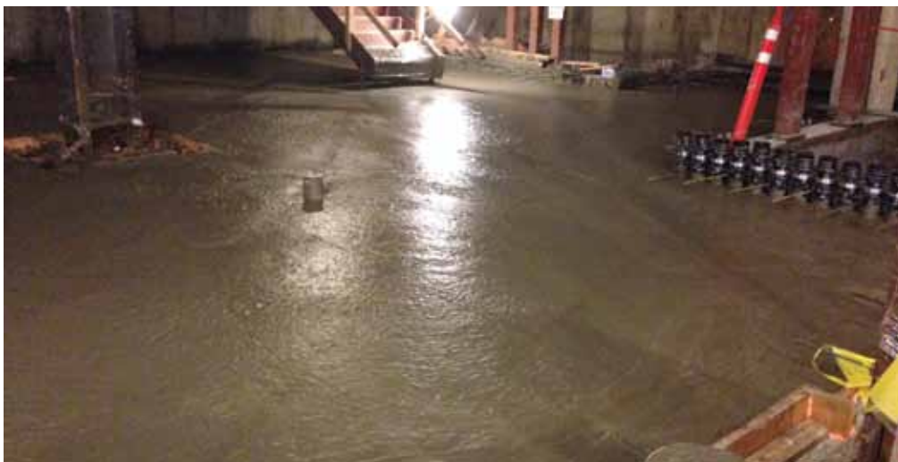
Large volumes in congested areas and difficult access are easy with cellular concrete. Shown is an 18-inch deep utility fill in San Francisco.
