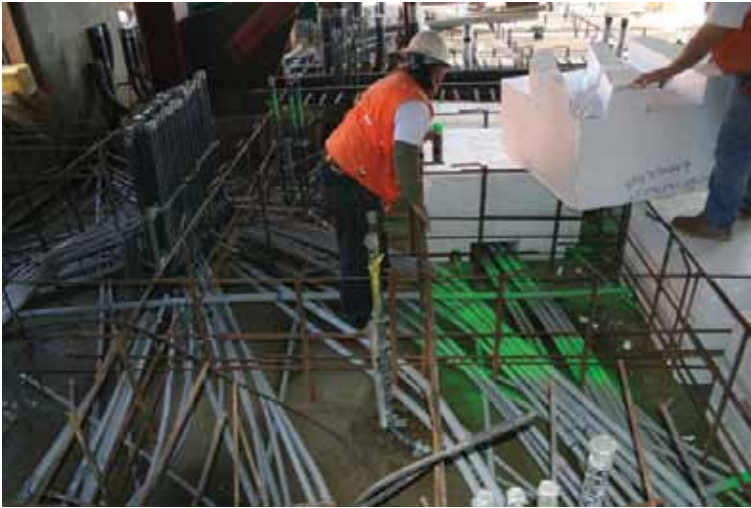
Too many Pipes! Using a lightweight flowable product saved significant time and labor.
