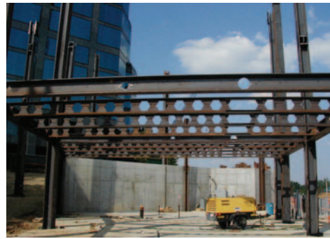
Castellated beam framing provided for the cost effective design as well as provide a 15-inch structure depth with prefabricated holes for sprinkler mains.
