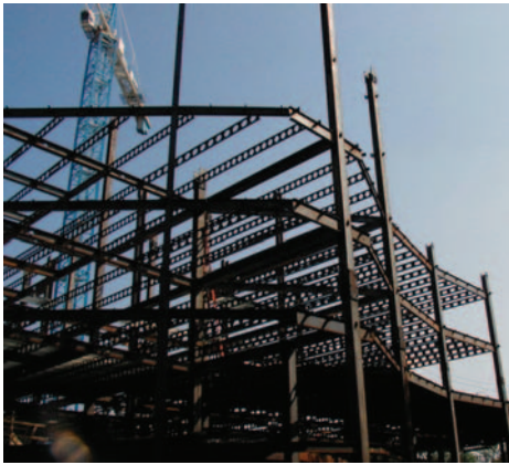
Difficult geometry with castellated beams create intense challenges to the structural design.
