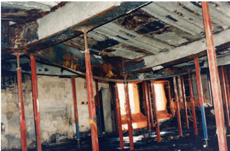
Deformed Floor (One Meridian Plaza)
