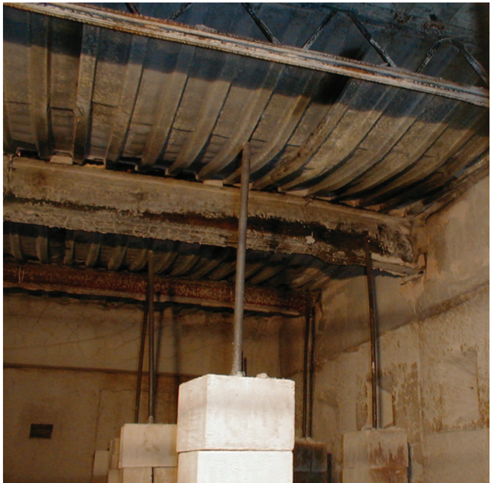
UL Assembly after Fire Test
