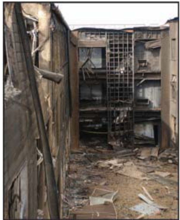
A wall of the E-Ring of the Pentagon leans inward and other walls show fire damage in this Sept. 14, 2001, photograph. Damage to the Pentagon was caused when the hijacked American Airlines flight slammed into the building on Sept. 11th. The terrorist attack caused extensive damage to the west face of the building and followed similar attacks on the twin towers of the World Trade Center in New York City. DoD photo by Staff Sgt. Larry A. Simmons, U.S. Air Force.
