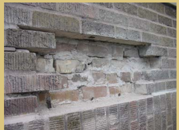
Figure 4: Corroded, perforated and failed metal strap ties in test opening
