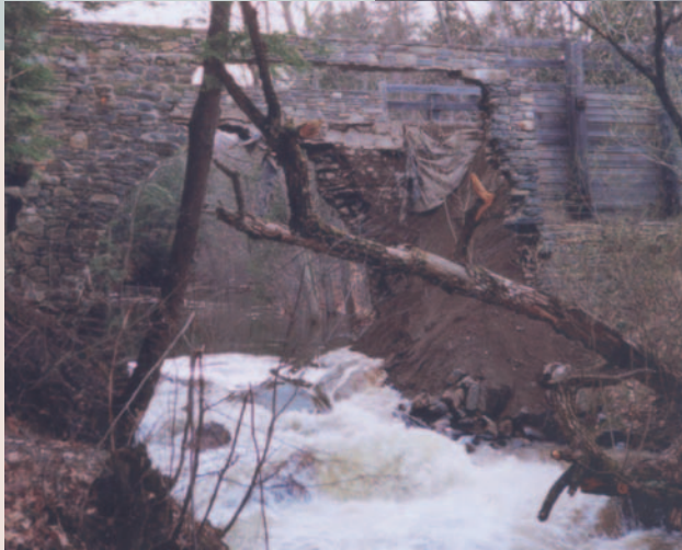
Malta stone arch, collapsed April 1993
