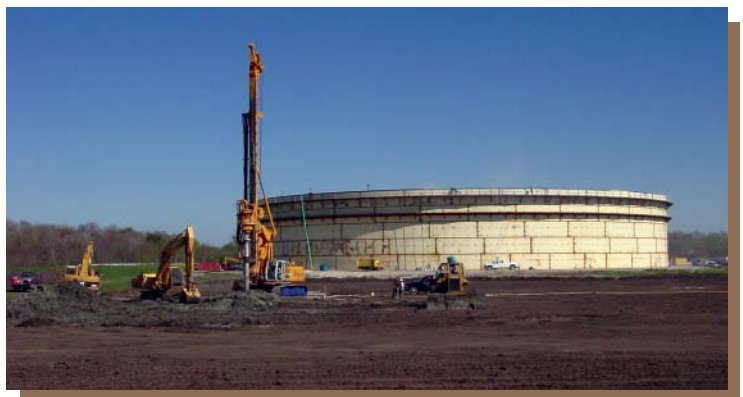
Figure 6: Soil Mixing reduced settlements and allowed construction of 310-foot diameter fuel oil storage tanks over soft soils.
