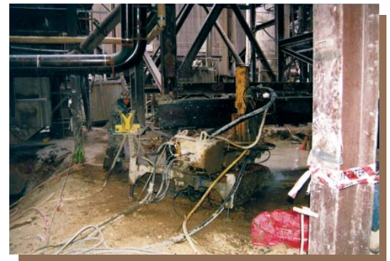
Figure 4: Jet Grouting next to an existing pile cap in restricted space at an operational power plant.
