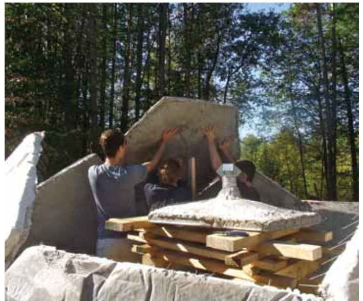
Figure 8. Second level panel supported and wired into place. Top panel with chimney supported by cribbing in the foreground. Courtesy of Megan Strand-Jordan.
