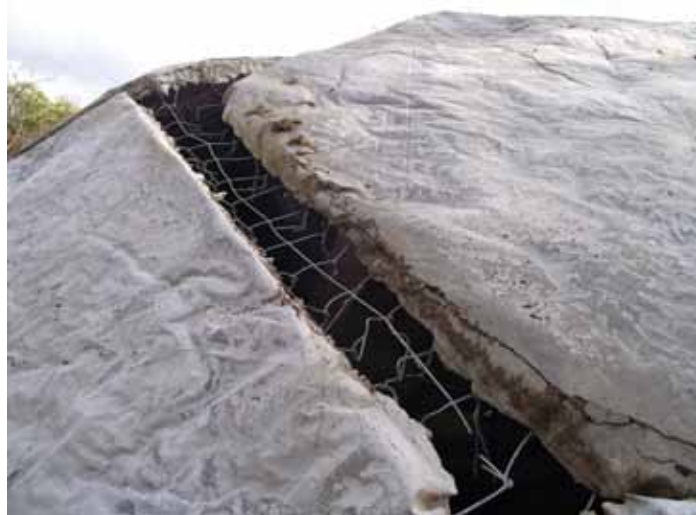
Figure 4. Attachments between the panels before addition of masonry between joints. Courtesy of Megan Strand-Jordan.
